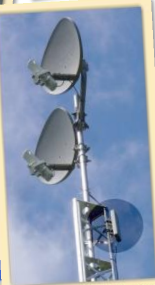
Two neighbours share the cost of a tower. Note the dark circle. This is a wireless bridge feeding the more distant neighbour. These devices connect neighbours, barns in-laws, offices etc. etc. Ask us.
